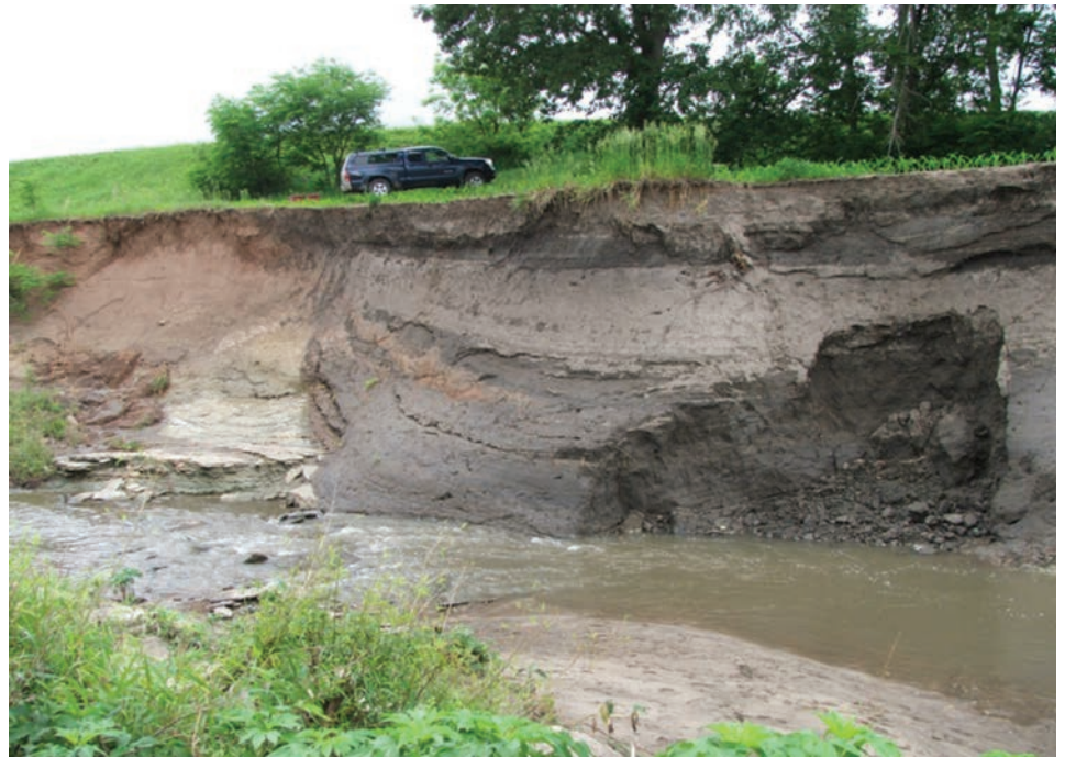
Figure 9. North Branch of the Black Vermillion River near Frankfort. These streams have been channelized to prevent flooding. This man-made action has caused the water to accelerate down the stream, cutting into the bank and incising the stream. The banks are so high that they are currently collapsing into the stream and will eventually create a new flood plane at a lower elevation. In the meantime, millions of tons of sediment are washing out of the river into Tuttle Creek Reservoir, impairing its ability to store water. (Photo courtesy of Phil Barnes.)
