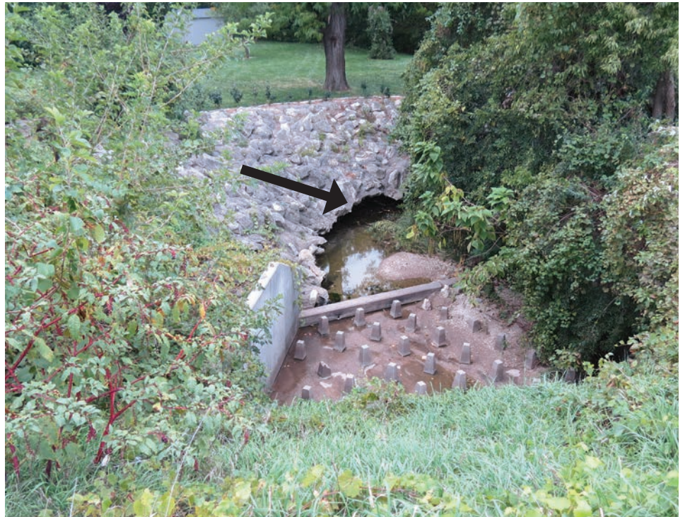
Figure 10. Downstream side of a concrete road culvert with a steep slope chute that carries water from a watershed area developed with shopping malls, businesses and residential housing area and the accompanying impervious areas of streets, parking lots and roof tops. The small concrete pillars are to help dissipate water energy. However, stream bank erosion was still occurring, resulting in the construction of a fortified stream bank. Notice that the fortification is being undercut (see arrow), which will eventually result in the structure's failure. (Photo courtesy of Danny H. Rogers.)
