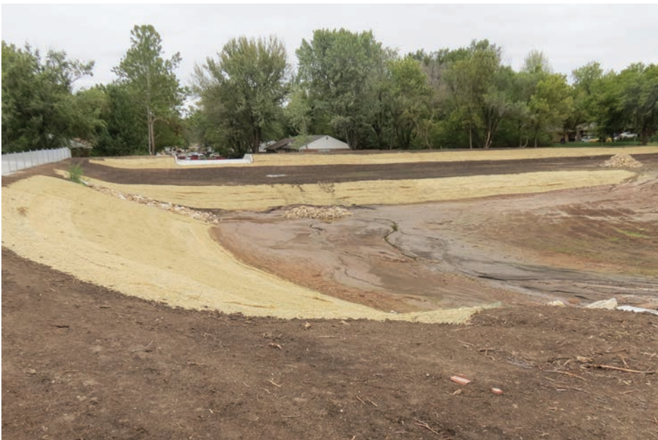
Figure 12. A nearly completed retention pond that receives water from a large apartment complex, sports facilities, and parking lots. The retention pond directs runoff water into a newly installed underground drainage pipe system and limits surface flow into the streets of a residential area. This pond has two outlets; one in the bottom of the pond and another that is located about halfway up the dam. The dam also has an emergency spillway to protect the structure in an extreme event. (Photo courtesy of Danny H. Rogers.)
