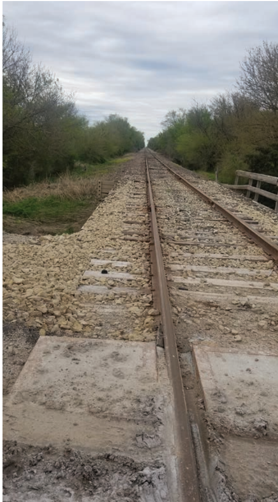
Figure 12. Vegetation control in railroad ballasts preserves ties and track stability. Photo: Frannie Miller
