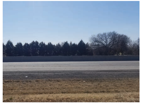
Figure 2. Weeds grow in median barriers built to prevent vehicles from crossing into oncoming traffic. Photo credit: Frannie Miller
