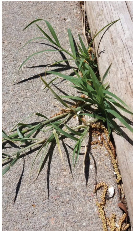
Figure 6. Cracks and crevices support roadside vegetation. Photo credit: Frannie Miller
