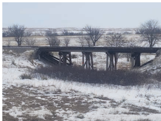
Figure 11. Vegetation around wooden bridges can be a serious fire hazard. Photo: Frannie Miller
