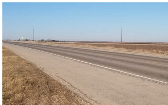
Figure 5. A road shoulder should be kept free of vegetation. Photo credit: Frannie Miller
