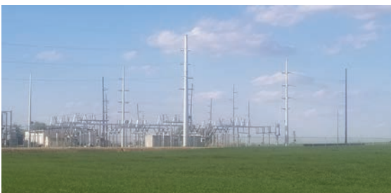
Figure 9. Substations are maintained and free of weeds for safety and aesthetics. Photo: Frannie Miller
