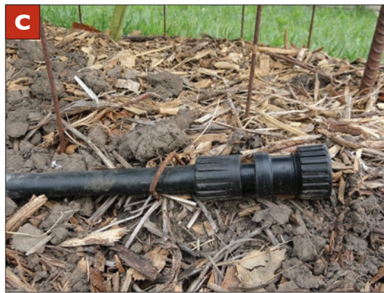
Figure 9. (A) A simple system for unrolling drip tape that can be used by a single installer. (B) Drip tape is connected to the header pipe with PVC connectors that have reverse-threaded locking collars. (C) Drip tubing is terminated with a premanufactured cap.
