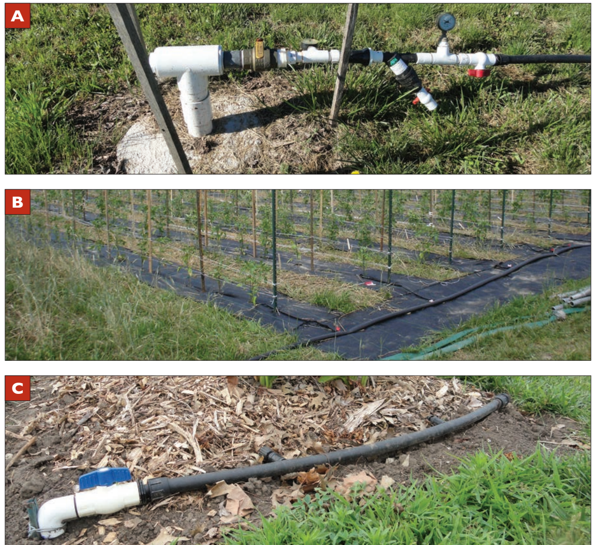
Figure 7. (A) Header pipe (left to right) with 1-inch pressure regulator, screen filter, pressure gauge, and valve connect to 1-inch poly piping. (B) Header pipe runs perpendicular to rows and distributes water to drip tape in a low-pressure drip system. Fabric mulch can be used to reduce weeds and grass growth under the header pipe. (C) Small/short header pipe is shown in a high-pressure system with a valve from underground piping.
