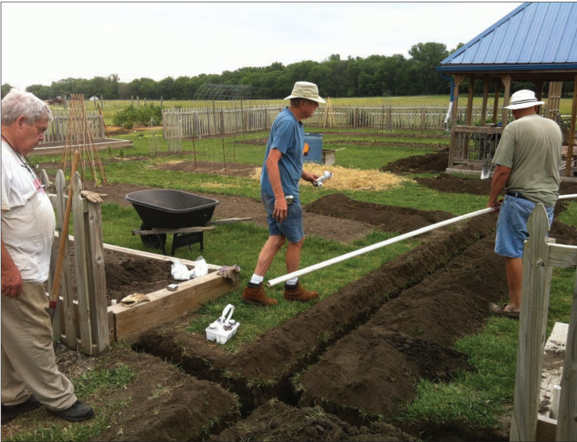
Figure 6. Distribution piping is installed belowground to move water to each bed where header pipes are installed.
