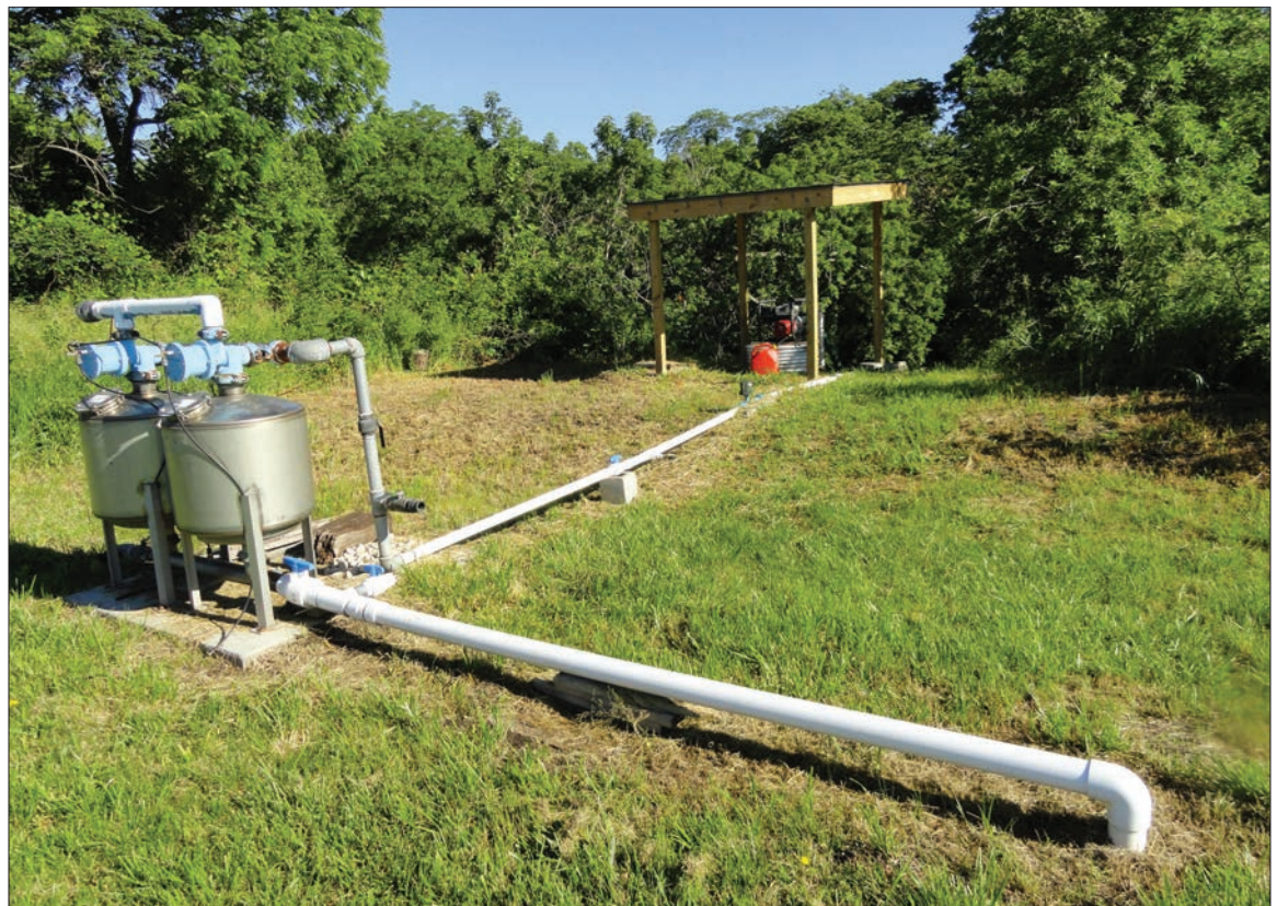
Figure 5. A sand filter (foreground) is used to filter creek water that is pumped with a gas-powered pump (background).
